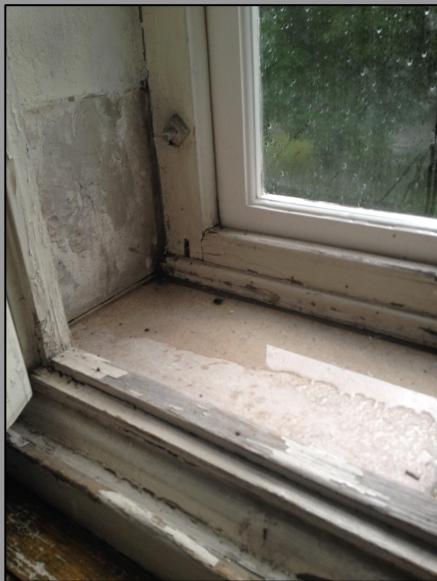
Water pooling in window sill after rain.
