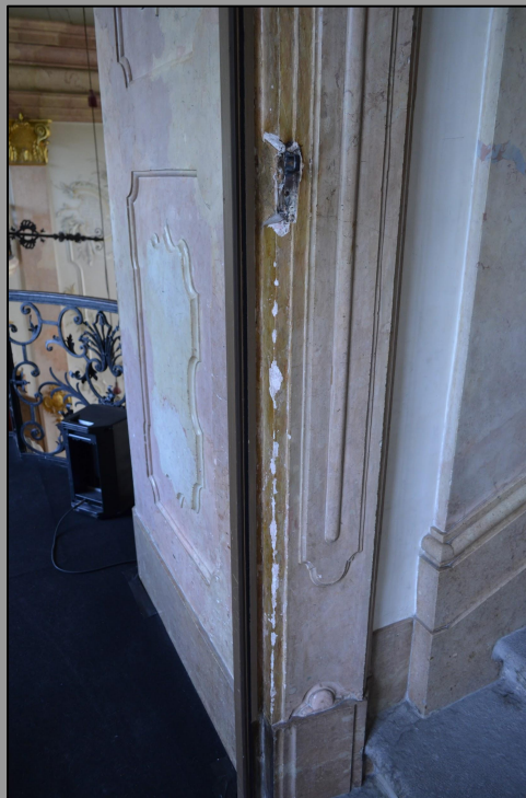
Damage to doorframes and stairs
