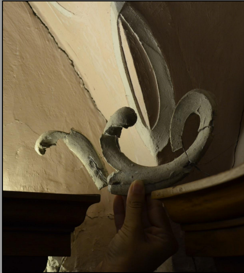
Broken stucco element from ceiling.
