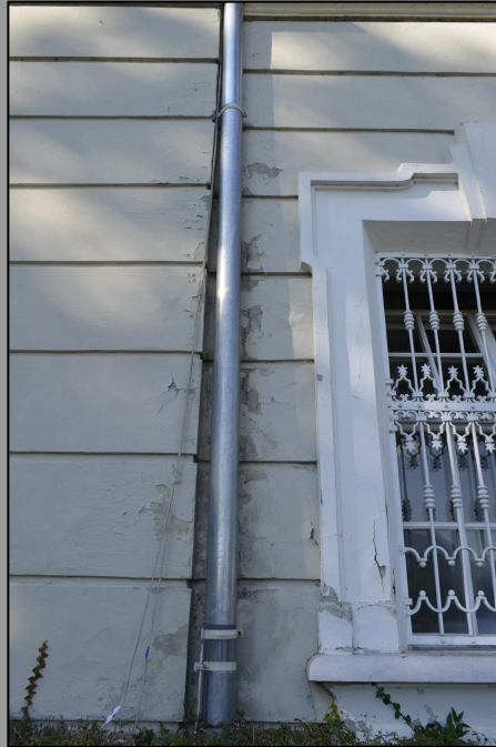
Exterior wall damaged near downspout.
